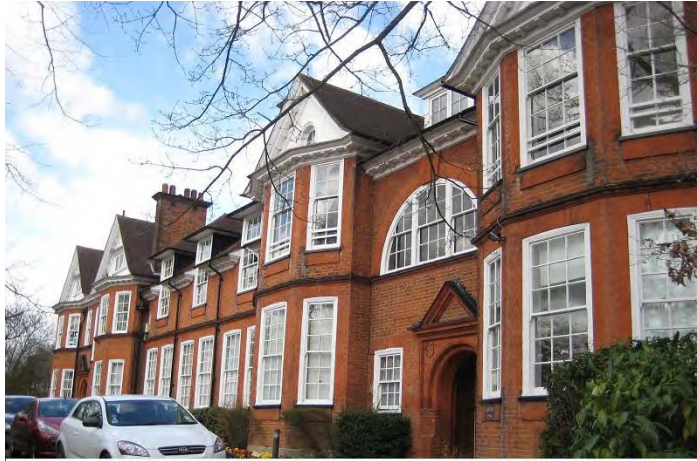
Picture 5.7 Original timber windows on Orley Farm School, South Hill Avenue, Harrow on the Hill
